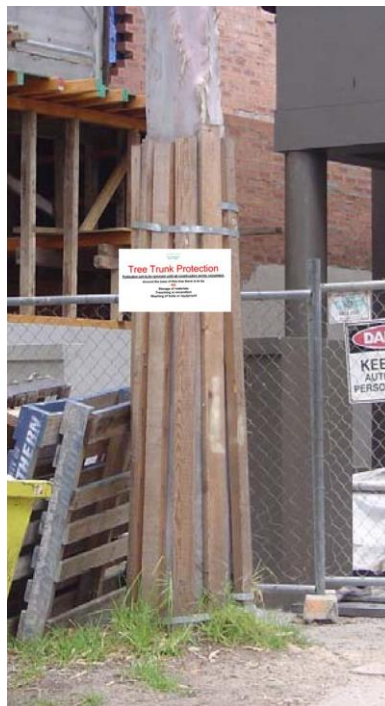
Image 1: Example of trunk protection with sign attached, recommended for Trees 78-81. P. Vezgoff.
